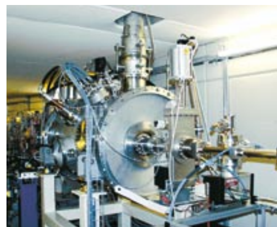
The superconducting cavity assembly as installed in the SLS storage ring.
