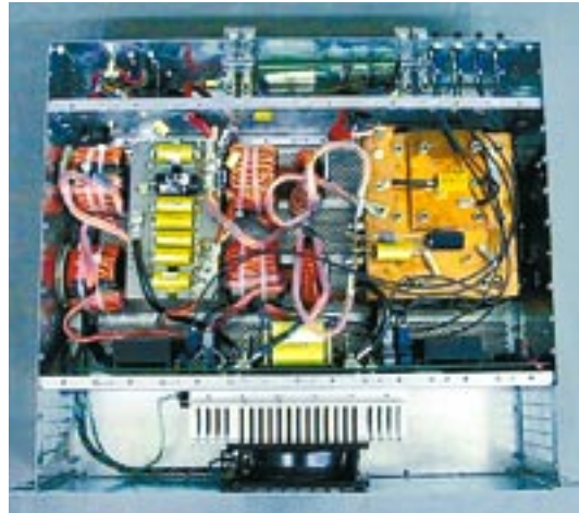
The power electronics of the kicker power supply.
