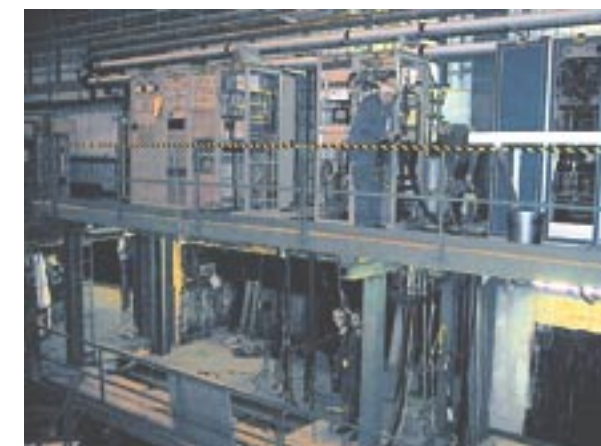
Changes afoot in the NA Hall: The existing electrical cabinets being removed.
