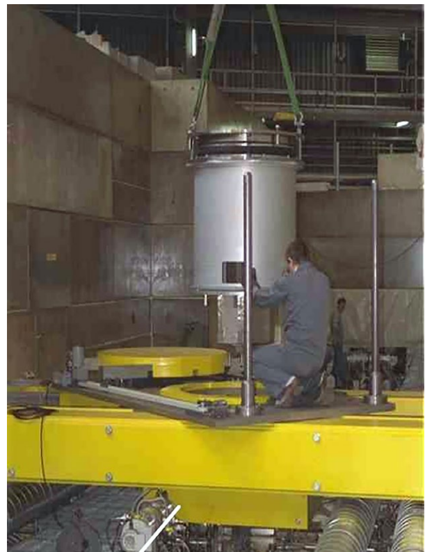
Figure 18.9: Installation of the contamination protection on the so-called bridge, where later the exchange flask will be positioned.
