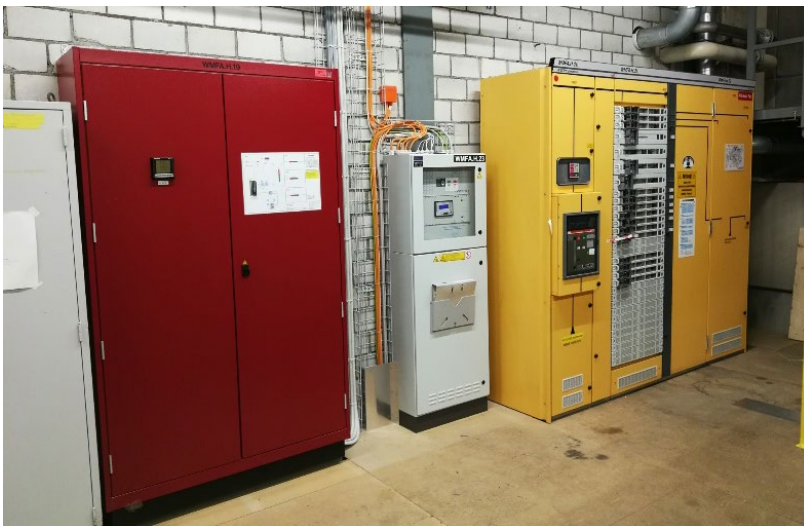
Figure 22.14: Electrical installations of UCN to be moved to WMFA.
