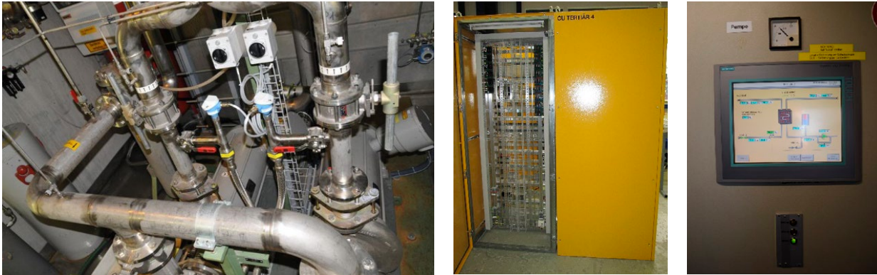
Figure 22.11: Components of the «Tertiär 4» cooling loop that will be reused for TATOOS.
