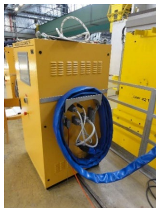
Figure 9.39: Control unit of the exchange flask side view.
