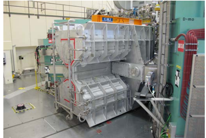
Figure 2: The new 50 MHz resonator installed in the Injector 2 cyclotron. The new resonator is capable of providing up to 400 kV/p accelerating voltage.
