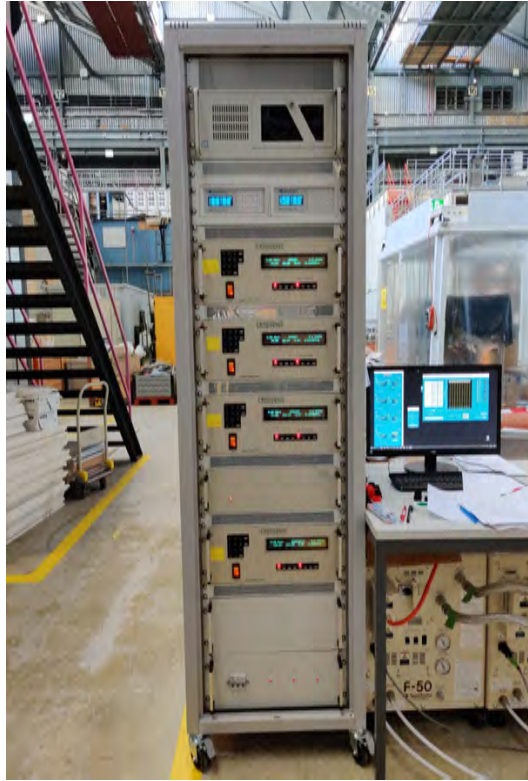
Figure 3.2: Electronics rack of the Mu3e magnet. From top to bottom: Dedicated computer, temperature monitor, power supplies for shim 2, shim 1, compensation and main coil.
