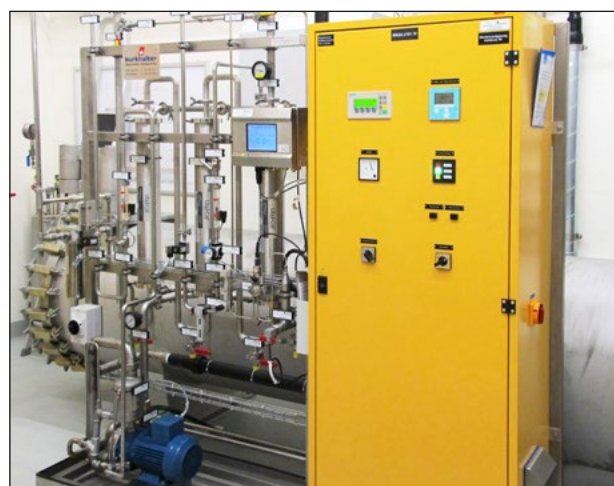
Figure 4: Degassing unit for the cooling circuits of the COMET cyclotron.
