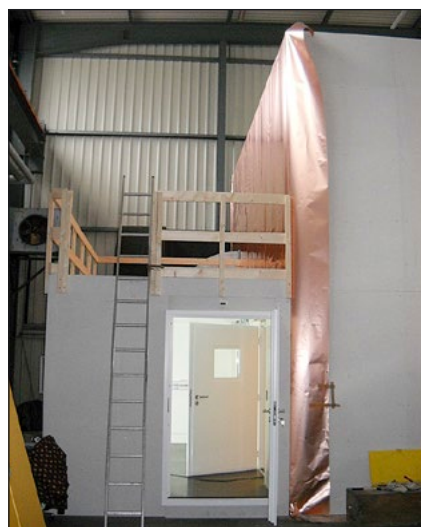
Figure 4: View of the entrance to the new n2EDM staging area in the WWHA hall, with the copper RF shielding already partially installed.
