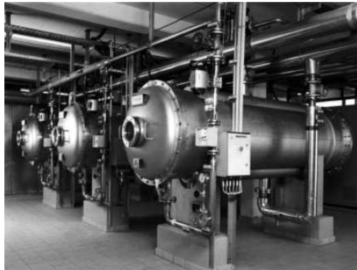
Figure 5.3: Ozone generators for the treatment of water [159].
