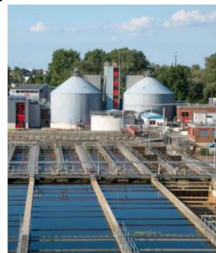
Municipal WWTP Morgenthal (SG) © morgenthal.ch
