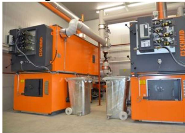
Autom. wood combustion CHP in Felben-Wellhausen (TG) © Schmid
